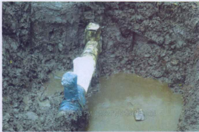
Figure 2: Wrapped Nipple on the pipeline.
